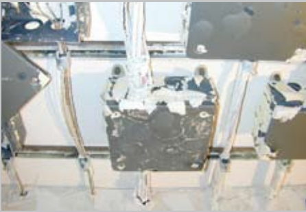
Junction box with connected cables after testing.
